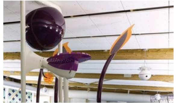
b. QuietSpace® Panels with gaps to keep the roof cavity well-ventilated
