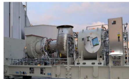
Gas turbine engine package
