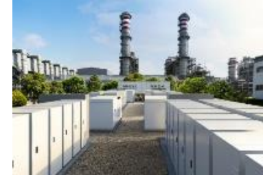
Power storage from batteries
