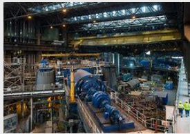
STEAM TURBINE: Performance, Mechanical, Gland Steam
