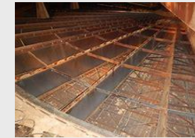
AIRHEATERS: Process, Mechanical
