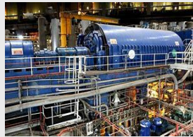
GENERATOR: Mechanical, Stator Cooling, Hydrogen, Oil Seals
