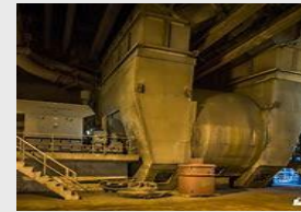
PA, FD, ID, BOFA Fans: Process, Mechanical, Motor Thermal
