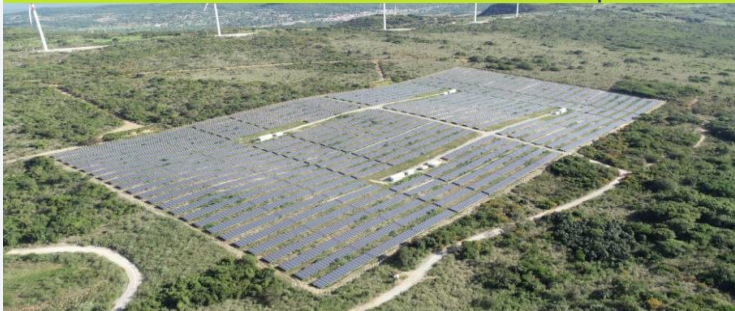
Fontes Solar – 16 ha – 11,01MWp
