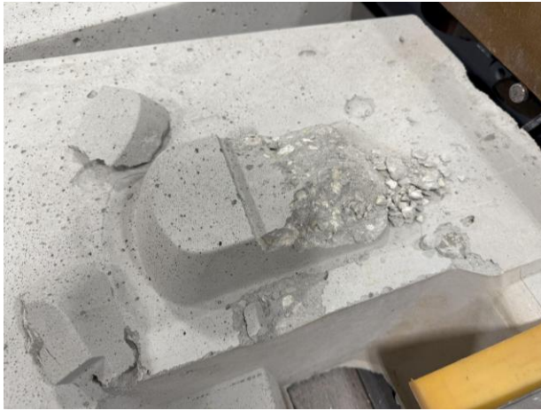
Figure 3 – Broken shear knob
