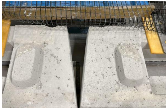
Figure 5 – Broken shear knobs
