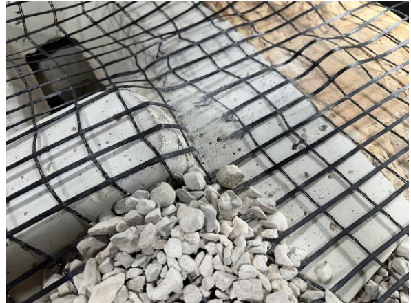
Figure 4 – Geogrid elongation and rupture
