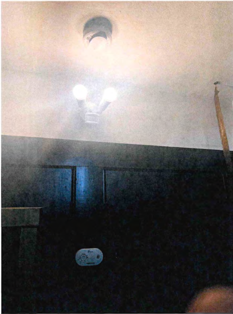
Smoke detectors and Carbon Monoxide Detectors
