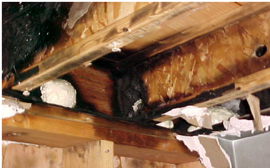
Example of Fire Damaged Engineered Wood Products
