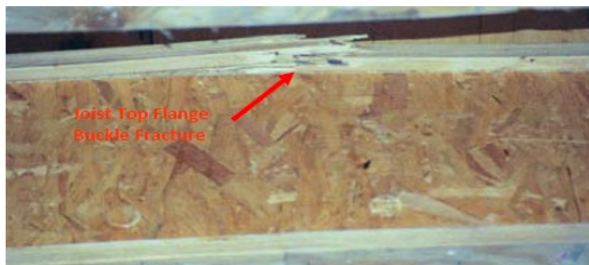
Figure 5: Example of I-Joist Failure Due to Improper Flange Bracing
